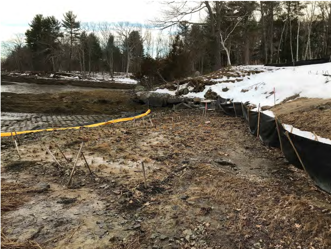
Fig 4: Toe of the slope and salt marsh restoration at the Eversource property/west side of the bay. Viewing south. (02-24-21)
