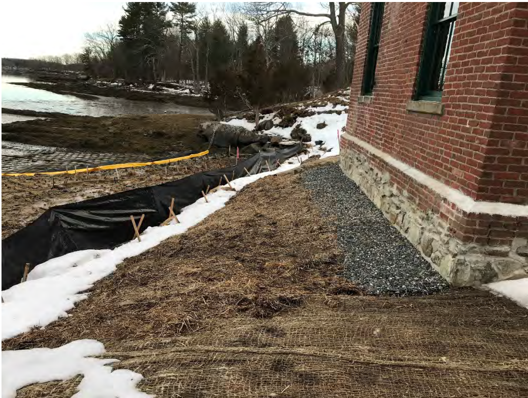
Fig 2: Slope between the cable house and salt marsh restoration at the Eversource property/west side of the bay. Viewing south. (02-24-21)
